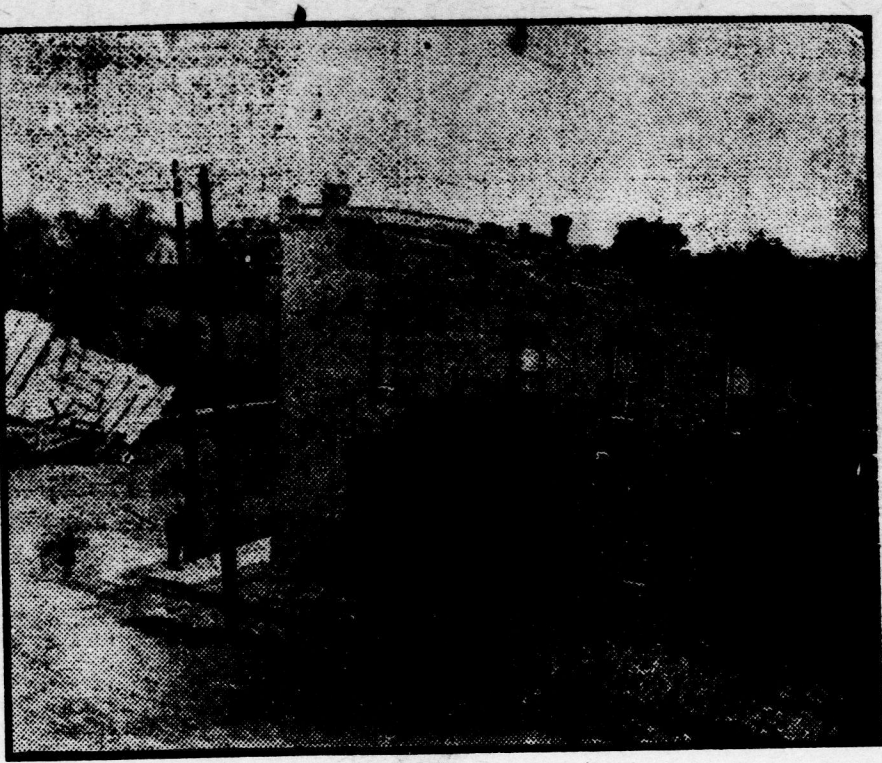
Friday's Storm at Rodney—View of the Rodney House, Which Was Unroofed and Otherwise Damaged.
