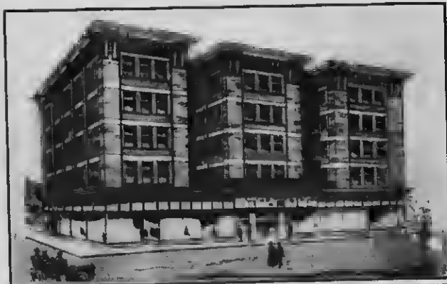
APARTMENT HOUSE, CORNER OF DUNSMUIR & RICHARDS STREETS Under construction by David Gibb & Son
