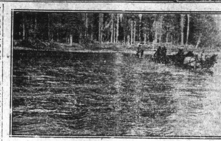
FORDING THE LITTLE SMOKY RIVER—Four horse stage, driven by J. Foreman McKay put in 2,200 feet of corduroy, just north of the Little Smoky river and 750 feet of corduroy four miles south of the Tony river. Foreman Johnson has put in about 2,000 feet of corduroy near Edson.
