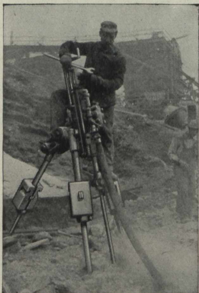
Hollow Piston Drill at work. Note cloud of cuttings ejected from hole.
