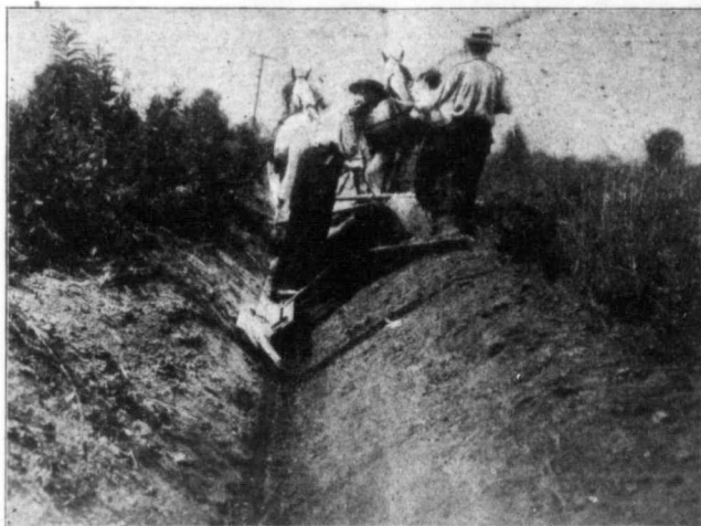
A V-bottom ditch will not cave in and carries perfectly either a large or small stream
