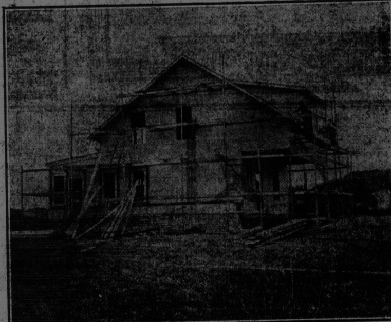
House being constructed at Glen Falls for Charles K. Cowan of M. R. A., Ltd., and which will be completed about May 1st
