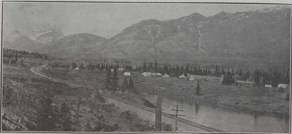
Part of Construction Camp, Looking West, Showing Location With Respect to the C.P.R. A Siding Leading to the Site May be Seen in the Background.
