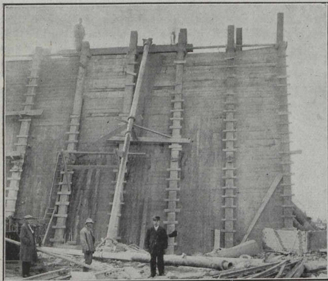
Pouring Dam, Montreal Water and Power Co. Length of Conveyer Stand-pipe, 47 Feet.
