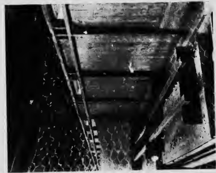
The openings, with shutters, at the back provide ventilation on hot nights
