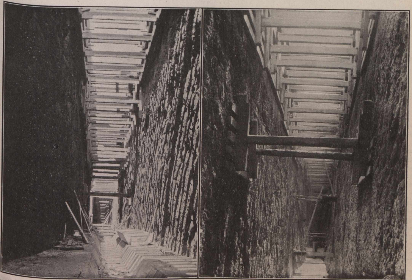
Fig. 1.—Trenching Methods, Delph Reservoir, Eng.—(Right) Rock Section Trench Bottom Ready for Concrete. (Left) Concrete Completed in Trench Bottom.
