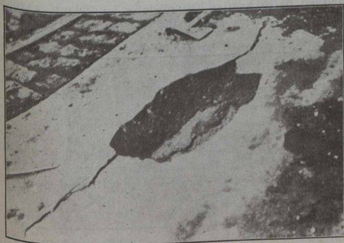
Showing Effect of Poor Drainage on Concrete Road.
