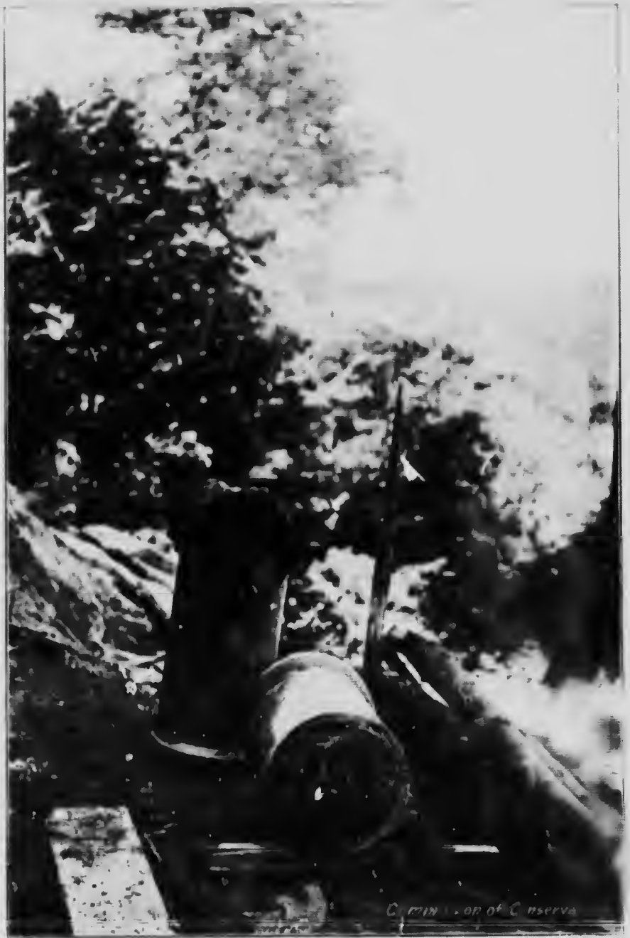
Example of Growth in Sewer Pipes
