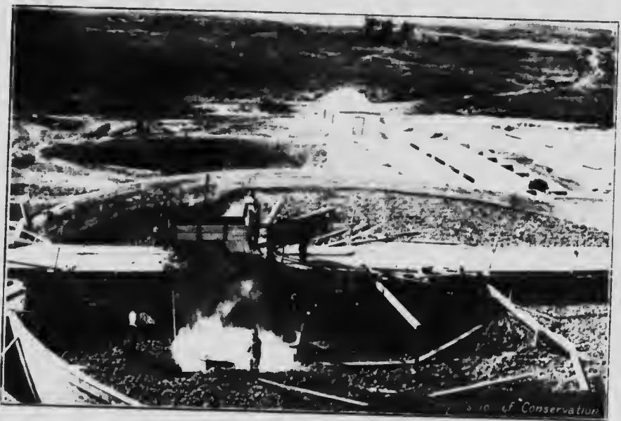
Same as Above Showing Method of Filling, Chlorinating House and Humus Tank in Background
