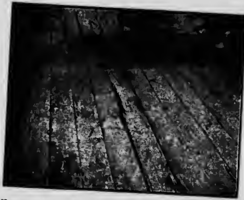
FIGURE 18.—A Floor that is difficult to keep clean.
