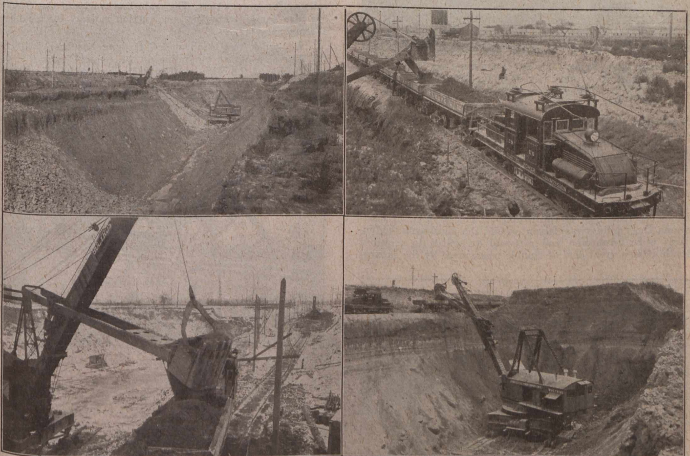
FOUR VIEWS OF ONE OF THE 8-YD. SHOVELS WORKING IN EARTH—TOP LEFT PHOTO SHOWS SOME RIP RAP IN PLACE—TOP RIGHT, TRAIN BEING LOADED AT STA. 346+81—BOTTOM LEFT, WORKING SOUTH OF THE WABASH R'Y—BOTTOM RIGHT, WORKING AGAINST A HIGH FACE AT STA. 346+81
