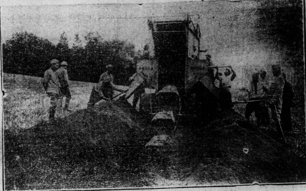
HOW THE FRENCH BUILD TRENCHES QUICKLY This photograph shows the famous French trench-builder at work. This picture shows the huge scoops which cut through earth and rock making a clean, clear-cut and immensely serviceable trench.
