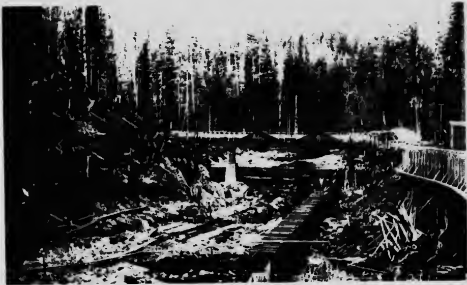
Vancouver Island Power Company Limited. Bridge carrying flume from Y Creek at junction with main flume prior to construction of Jordan River Storage Dam.
