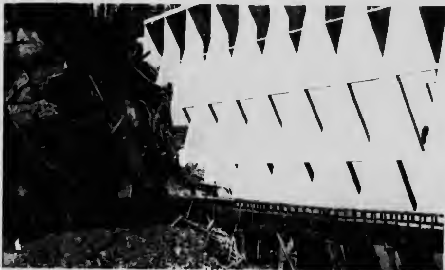
Vancouver Island Power Company Limited. West end of Jordan River Dam, showing buttresses and tie beams.
