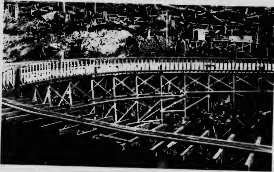
Vancouver Island Power Company Limited. Flume between Jordan River Dam and Forebay Reservoir.
