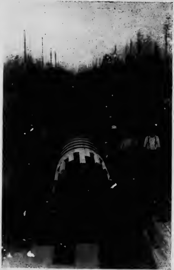
Canadian Collieries (Dunsmuir) Ltd. Wood Stave Pipe near Power House. End view.
