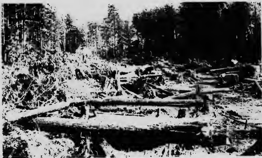
City of Prince Rupert-Woodworth Lake, near Prince Rupert. Clearing for Pole Line right-of-way.
