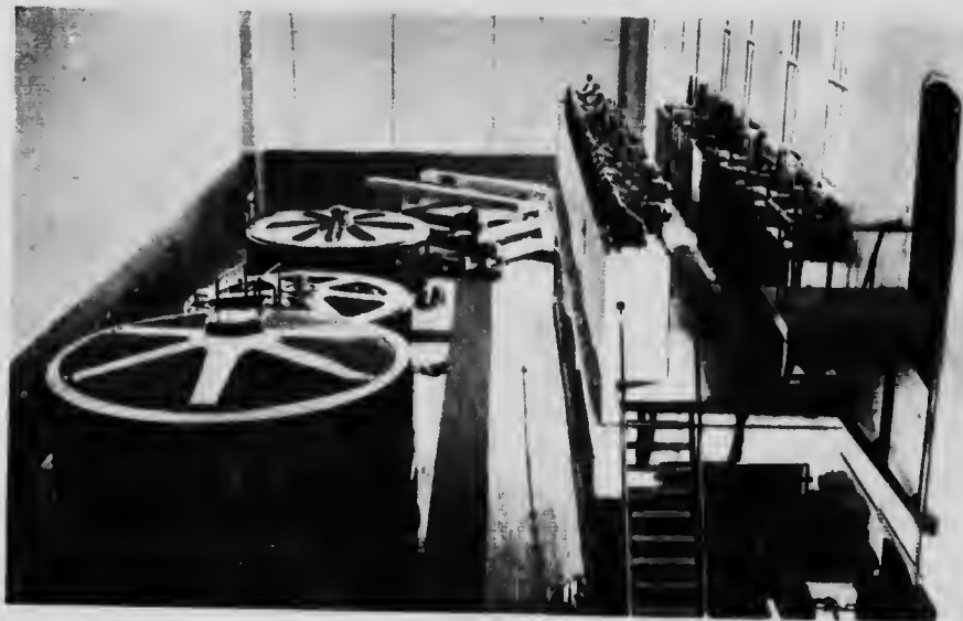
Kootenay River Development. Generator Room, No. 2 Plant, Upper Bonnington Falls.
