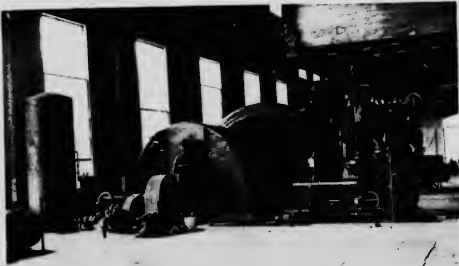
Vancouver Island Power Company Limited. No. 3 unit in position showing governors, oil pumps and gate valves.
