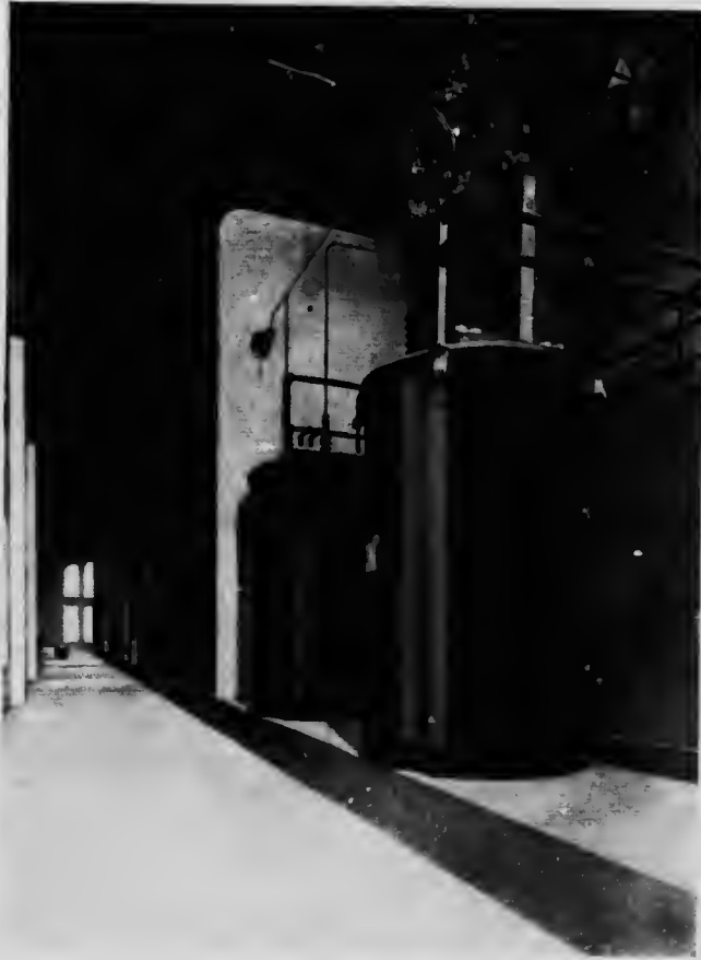
Coquillam-Bunizen Development. Transformer Room, Power House No. 2, Lake Buntzen.
