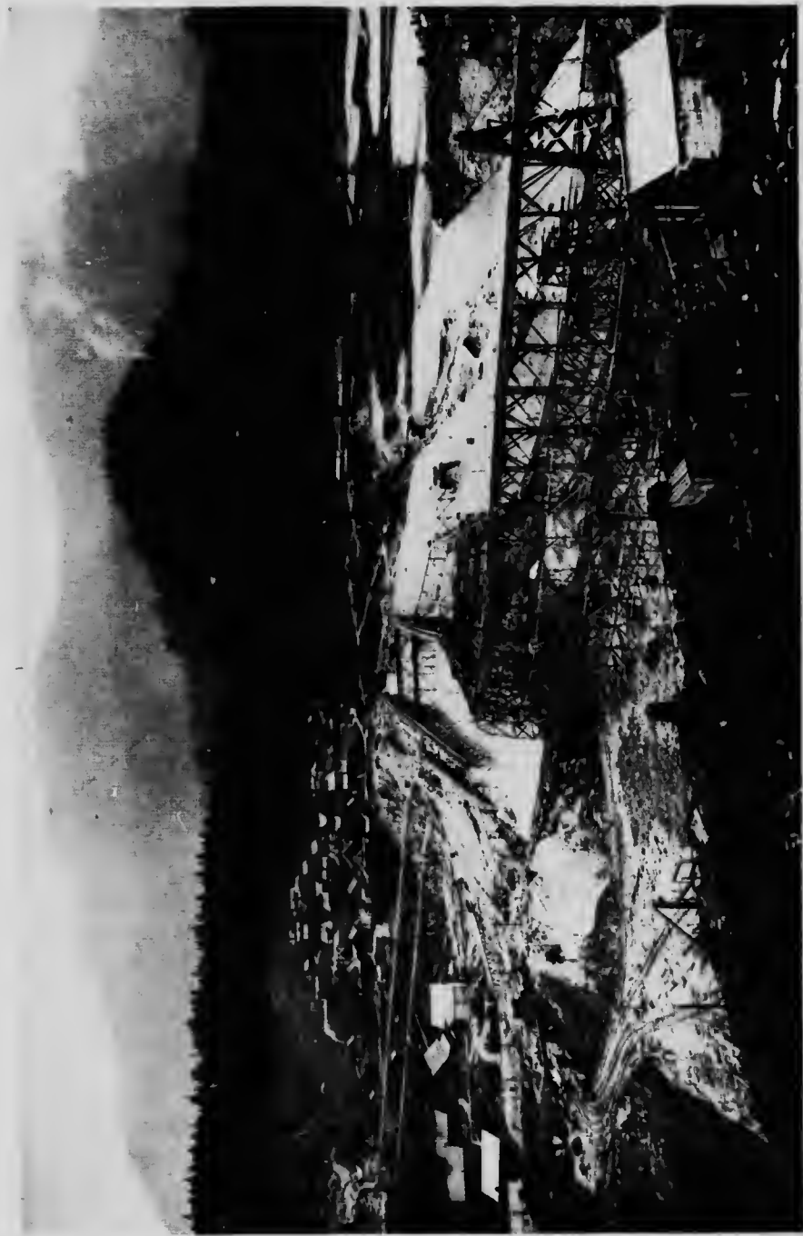
Coquitlam-Buntzen Development. View taken from East Side of spillway showing Coquitlam Dam in construction. The trestle work carries the flume.
