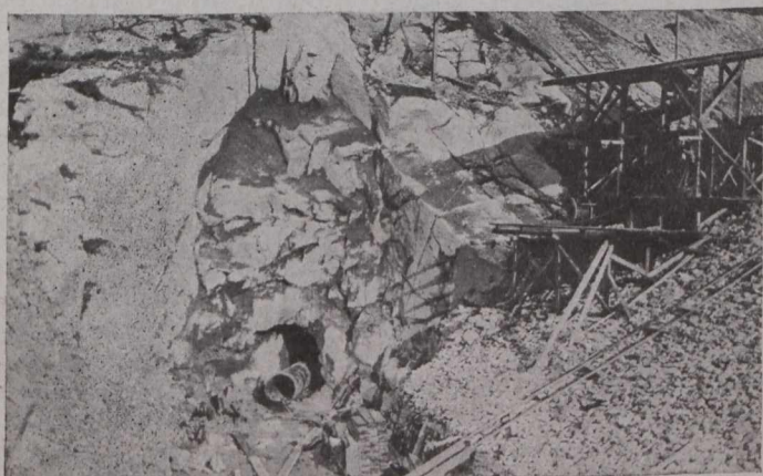
Fig. 5.—Foundation for Water Tower—4-ft. Pipe in Entrance of Tunnel. Note Solid Rock Foundation.
