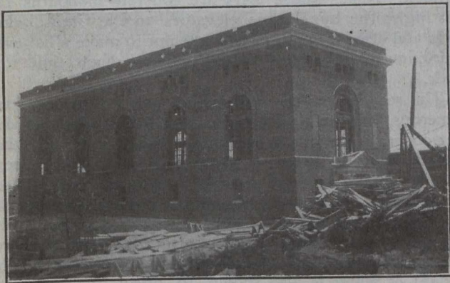
Fig. No. 5.—Pumping Plant at Lemieux Island
