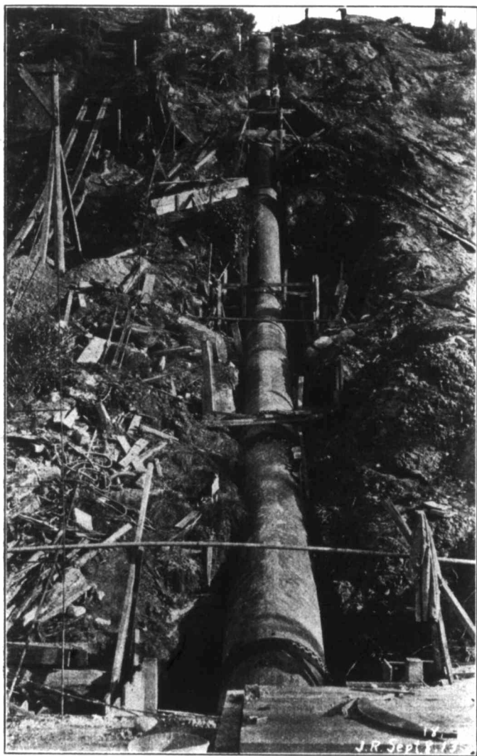
Fig. 9.—No. 3 Pipe Line.—View from power house.
