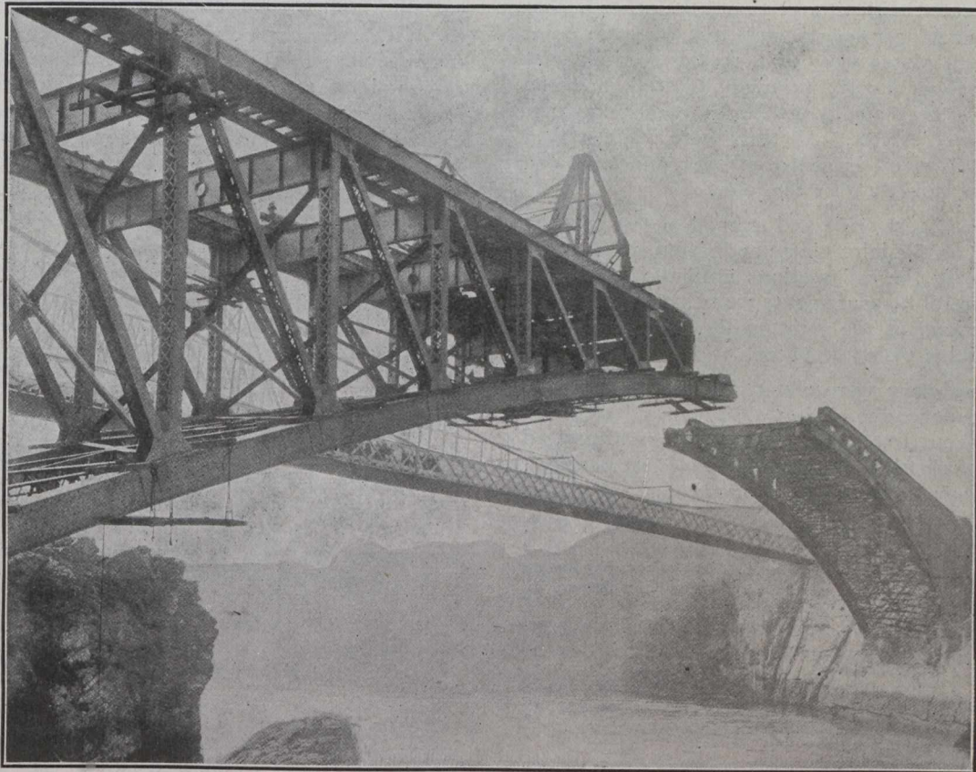
St. John Arch Highway Bridge, During Erection, to Replace the Old Suspension Span.
