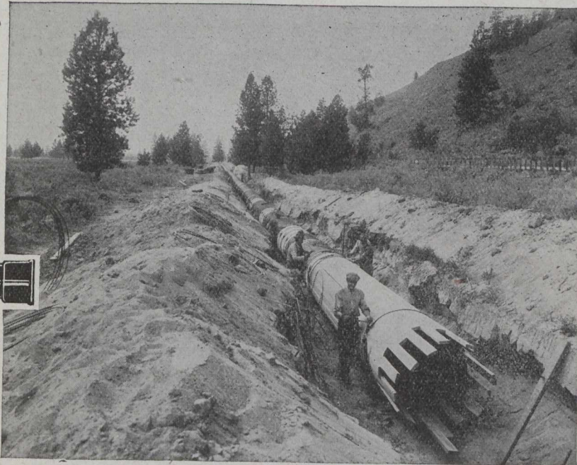
48 in. CONTINUOUS STAVE LINE.
