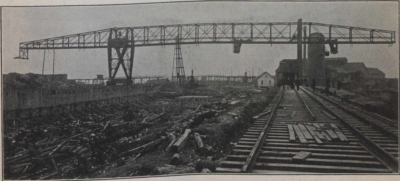
Fig. 1.—Part of the Piling Used for Carrying the Concrete Slab. Photograph taken April 5, or 15 Working Days after Excavation was Started.
