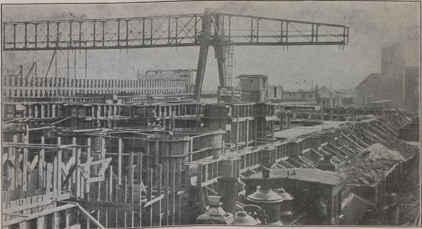
Fig. 5.—Showing by Height of the Locomotive the Large Amount of Form Work needed to give a Yard Level 16 Feet above Top of Piles.
