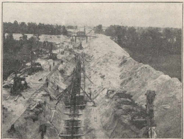
Bird's Eye View of Gary Sewer, Showing Pumping Plant, Trench, Clamshell, Backfilling and New Steel Plant in Far Distance.
