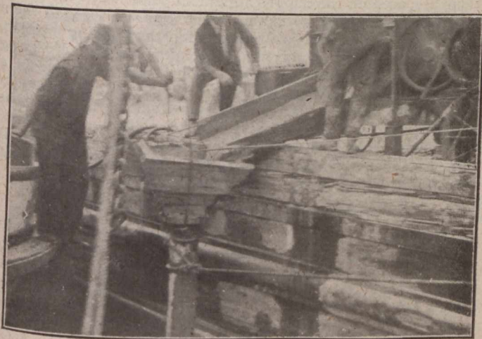
FIG. 6—CHUTING CONCRETE THROUGH 8-IN. PIPE TO INTAKE STRUCTURE 47 FT. BELOW WATER LEVEL
