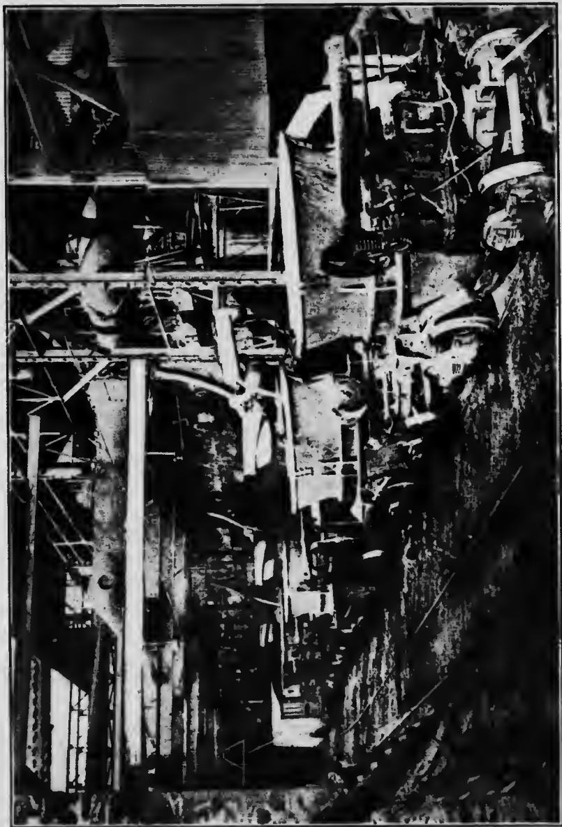
Interior of the blast furnace building, slag sile, British Columbia Copper Co., Greenwood, B.C.
