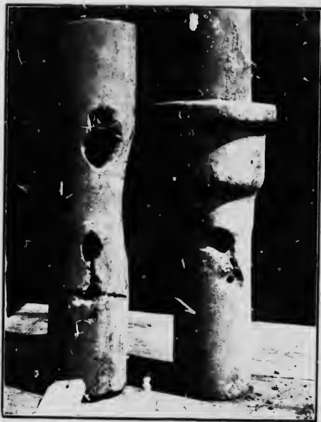
Fig. 1. Electrolytic Action on Water Mains.
