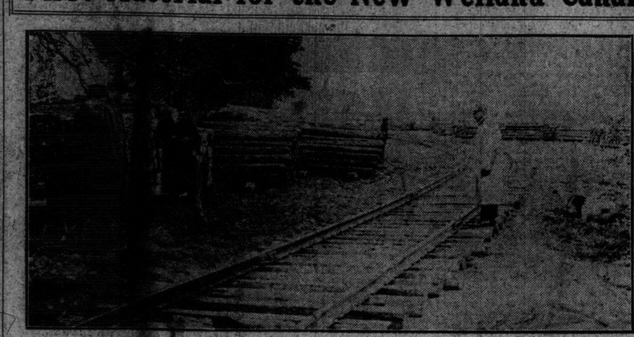
Ties and Timbers Brought into Port Weller Over a Spur Line From the New C.N.R. Electric Road From St. Catharines to Niagara-on-the-Lake.
