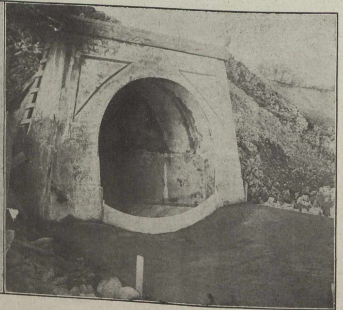
Fig. 7.—Outlet of Main Garrison Creek Storm Overflow Sewer at the Foot of Strachan Avenue.
