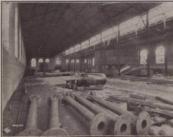
Fig. 7.—Interior of Filter House, Looking Towards the North, at Start of Tank Erection. Cast Iron Supporting Columns for Filters Shown in Foreground.
