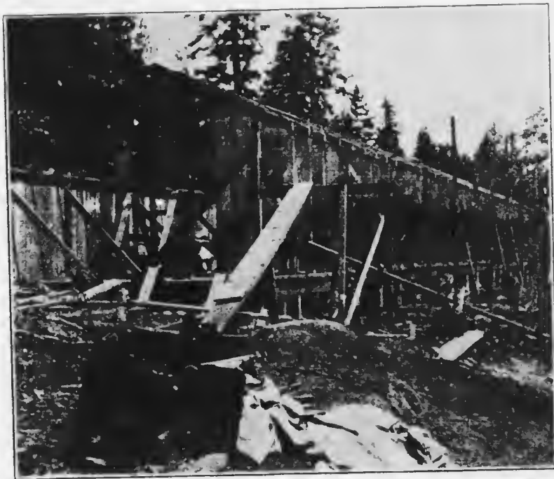
It is necessary to keep the house on a level plane. We would suggest the hire of a team, man, and scoop shovel for a day in such an instance to take the dirt from the slope and level the same to a certain extent.
