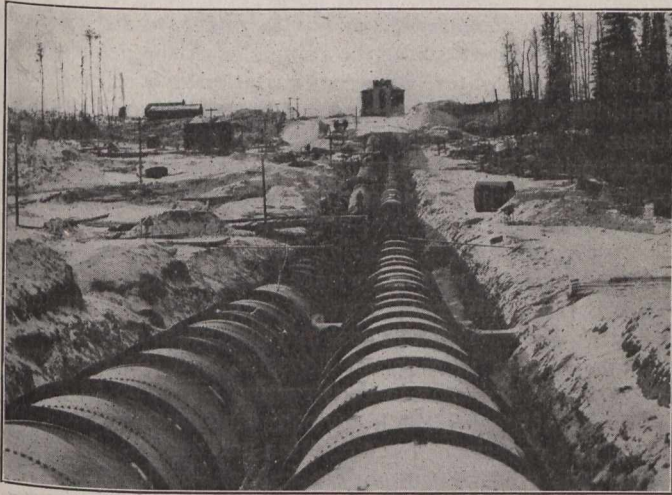
Two 8-ft. Iron Pipes, 1,300 ft. Long, from Surge Tank (in distance) to Power House at Wawaiten Falls.
