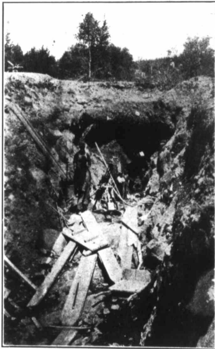
Open Cut at South Portal. Spoil going to Shaft to be Hoisted.
