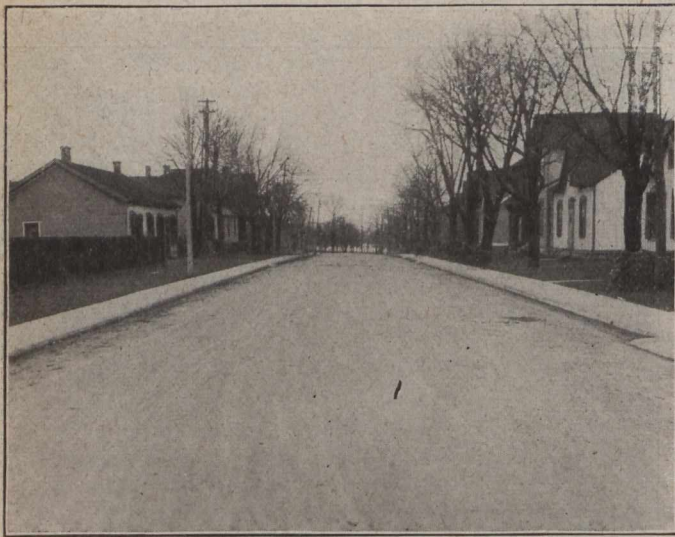
Devonport Street, Hamilton, macadam treated with asphalt road oil in early Spring, 1917. Photo in Fall after season's traffic
