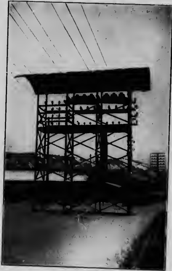
Fig. 4.—Junction Tower, Transmission Line.
