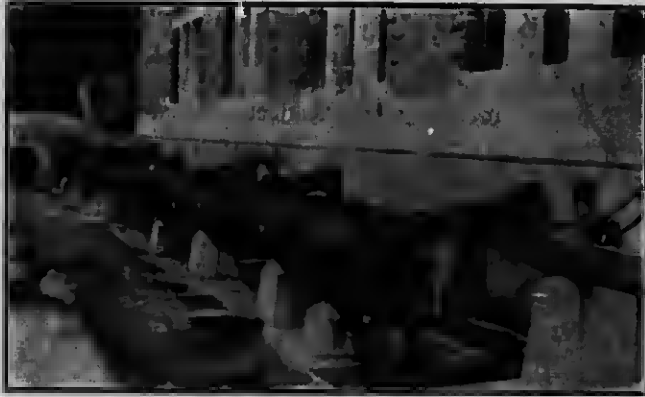
Fig. 11.—Engelberg: Penstock End and Its Distributor.
