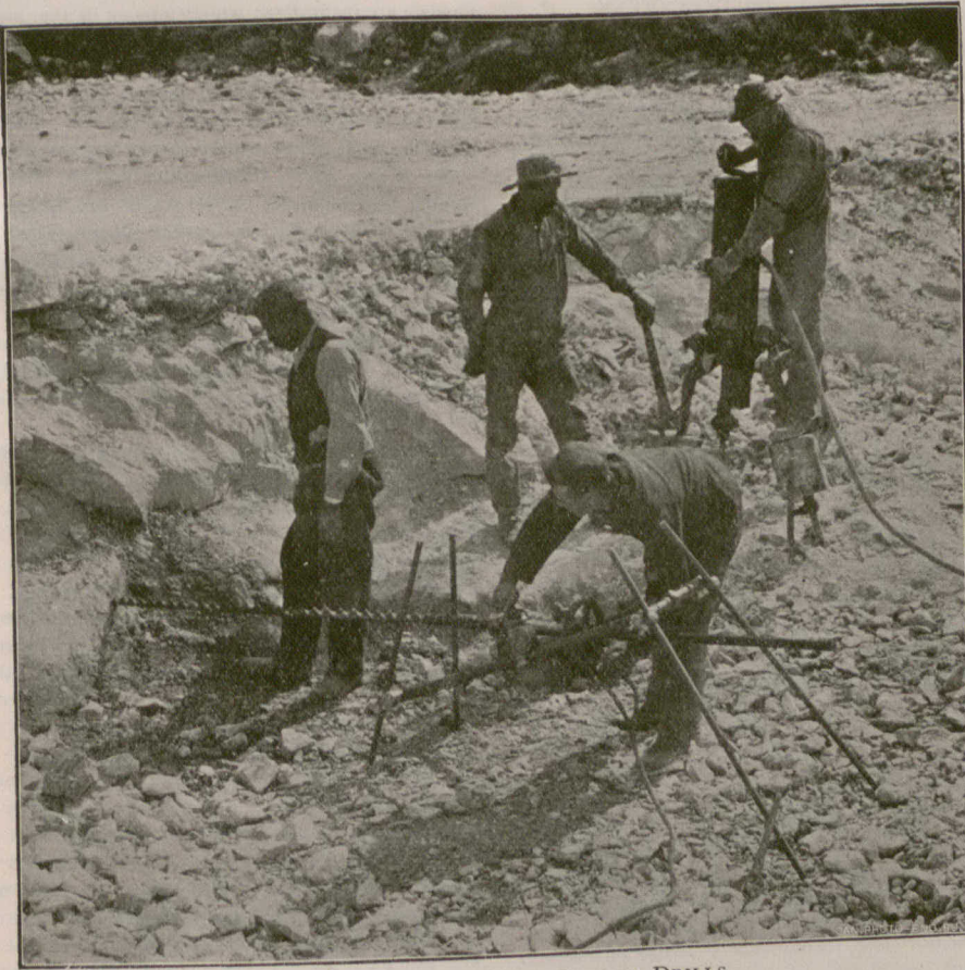
ELECTRIC PERCUSSION AND ROTARY DRILLS, IN OPERATION AT THE WINDSOR GYPSUM CO. S QUARRIES, WINDSOR, N. S.
