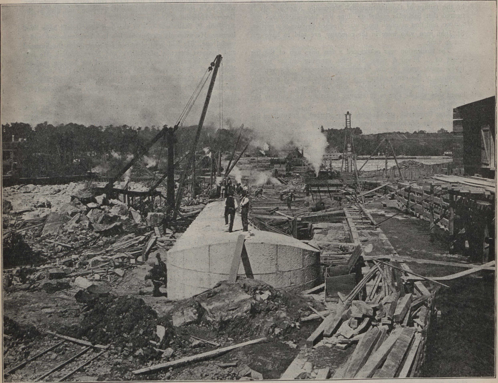
Bull-Nose of gathering dam. This dam which is of granite and concrete, will be entirely submerged but will act as a huge arm to draw the water into the wheel pit. The foaming rapids outside the present false work can be seen in the distance on the right.
