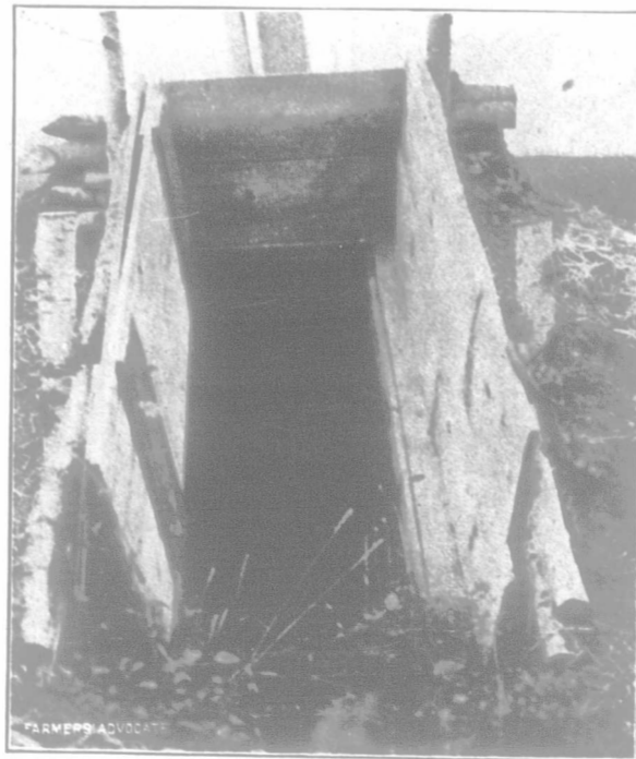
ENTRANCE TO UNDERGROUND ROOTHOUSE 5 FEET DEEP AND 50x20 FEET IN LENGTH AND WIDTH
