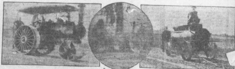
Up-to-date Machinery is Necessary for Economical County Road Construction. Snapped at Work Last Summer by the Farm and Dairy Camera. Left: A road roller at work in Oxford Co., Ont. Centre: Scraper for digging up old road beds, York Co., Ont. Right: Road sprinkler working ahead of the road roller, Oxford Co., Ont.
