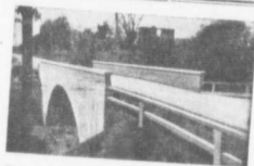
The type of permanent culverts universally used for road work.
