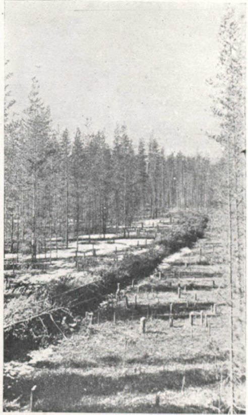
CUTTING A NEW ROAD IN BRITISH COLUMBIA Note how carefully the debris is piled for burning in the centre.
