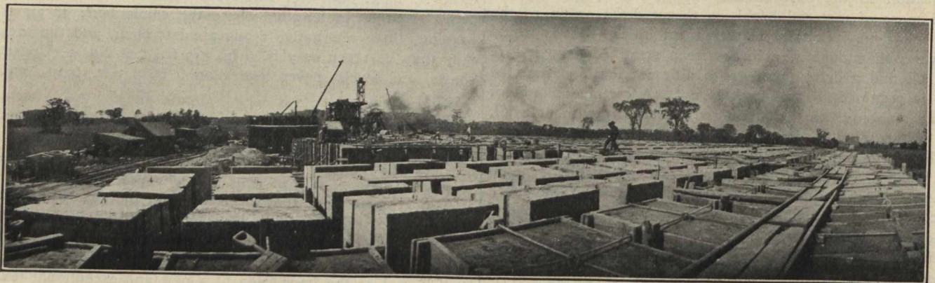
Making Concrete Footing Blocks for Tarte Pier, Showing Track for Trucks on Top of Blocks.
