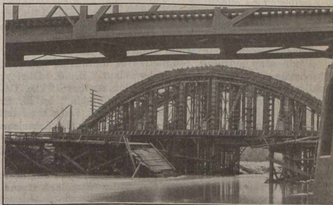
DAMAGE TO TEMPORARY TRESTLE AND CENTERING UNDER NEW CONCRETE BRIDGE CROSSING ETOBICOKE RIVER
