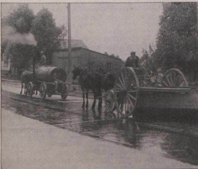
One of the methods of applying and spreading Dolarway Bitumen on Concrete Base.
