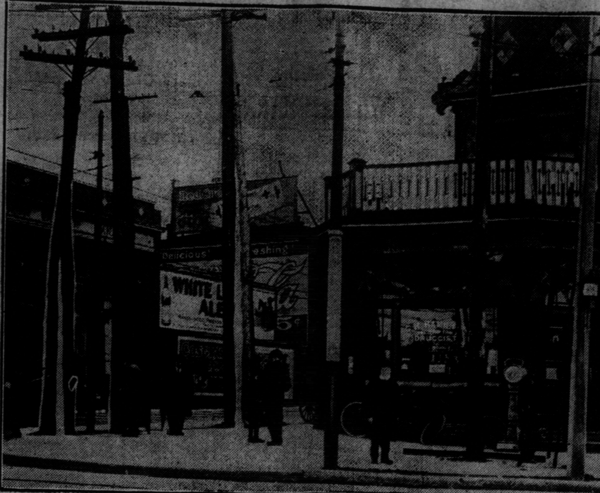
This photograph shows some of the poles at the junction of King and Queen streets at Sunnyside. Two or three more have been put up since the picture was taken.
