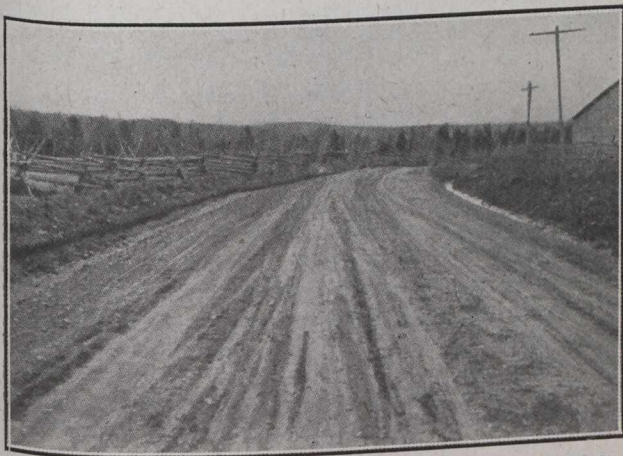
Main Port Road. A section of Earth Road which is still in splendid condition after being improved two years ago.
