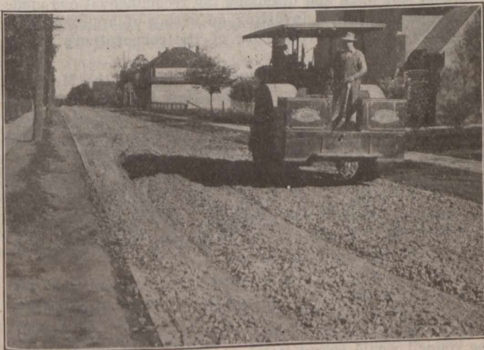
BROKEN STONE BASE FOR BITUMINOUS ROAD, PENETRATION TYPE, MIMICO, ONT., SHOWING DEPRESSED CURB
