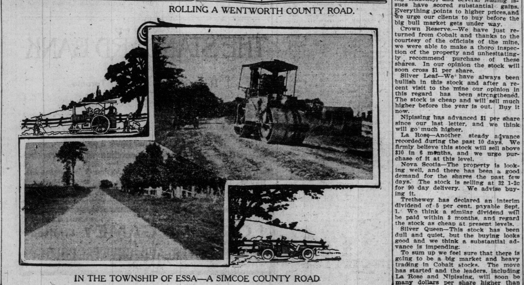
ROLLING A WENTWORTH COUNTY ROAD. IN THE TOWNSHIP OF ESSA—A SIMCOE COUNTY ROAD.
