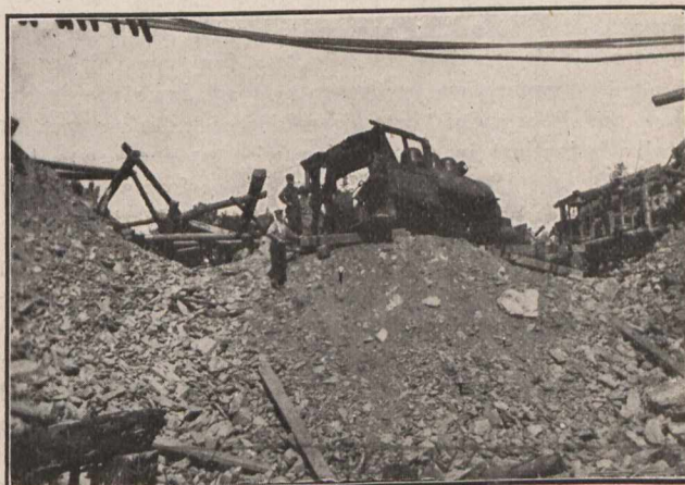
Trestle after the Collapse, showing Donkey Engine on Dump and Track Rails Suspended.
