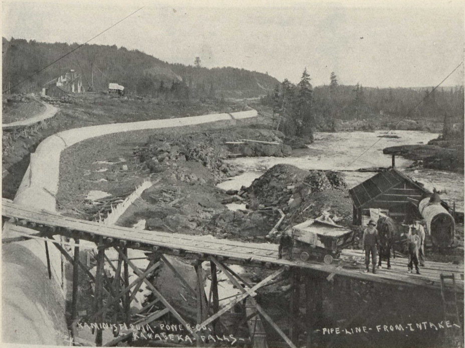
CONCRETE PIPE 10½ FEET IN DIAMETER LEADING FROM INTAKE TO FOREBAY OR RESERVOIR
