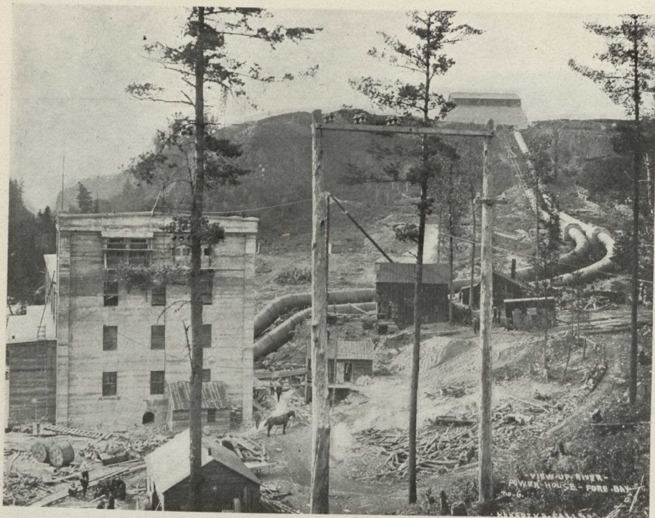
TWO SEVEN-FOOT PENSTOCKS FROM FOREBAY TO POWER HOUSE, 180 FEET OF HEAD
