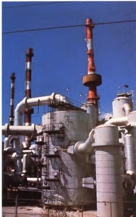
Noranda's CEZinc acid plant.
