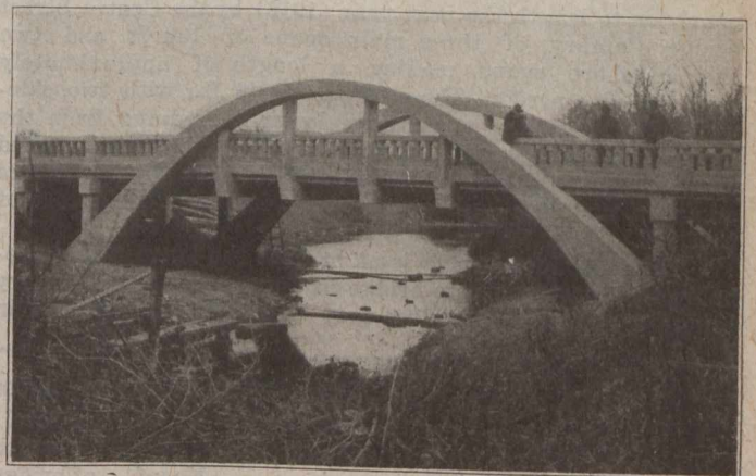
ARDEN ARCH NO. 3, MANITOBA (Open Spandrel Arch with Floor Suspended Midway Between Springings and Crown)
