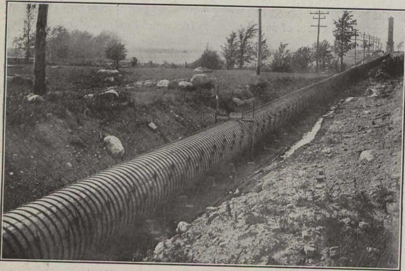
Fig. 8.—Wood-stave Pipe Line Leading to Surge Tank.
